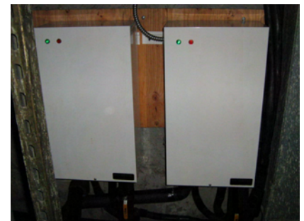
Two Enviro-Pak's generating hot water by recycling wasted heat from the refrigeration system.
