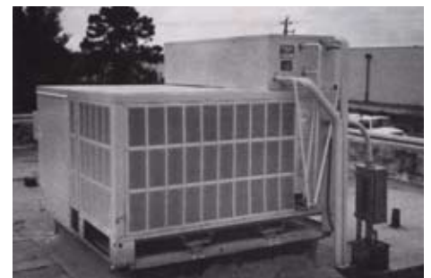
Enviro-Temp, on the rooftop, generating hot water by recycling wasted heat from the refrigeration system.
